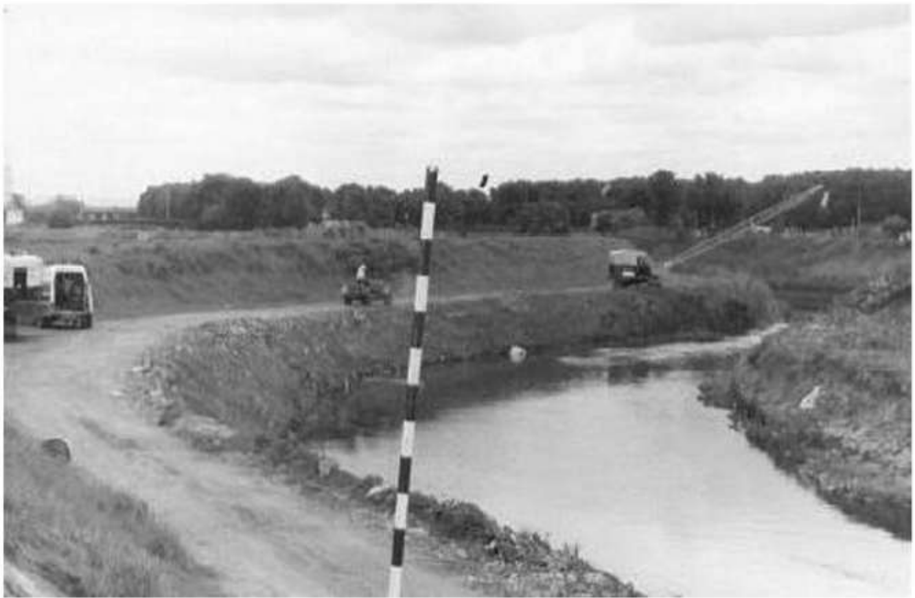
The Mersey Bank, Stretford, SJ7892/3, undergoing reconstruction in July 1987. Much high-quality habitat was lost in this process, but has since recovered. See page 13.
